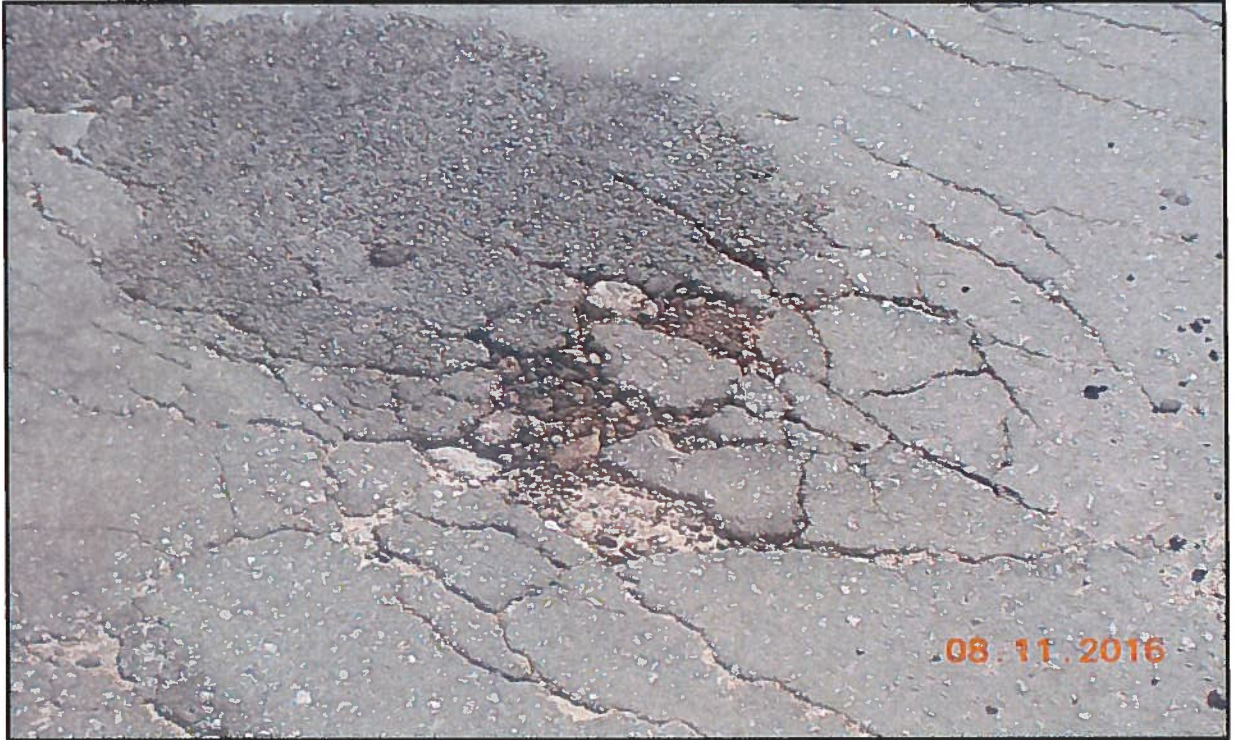
Photo 5: Loss of Bond & Map Cracking in Deck– Northwest Quadrant
