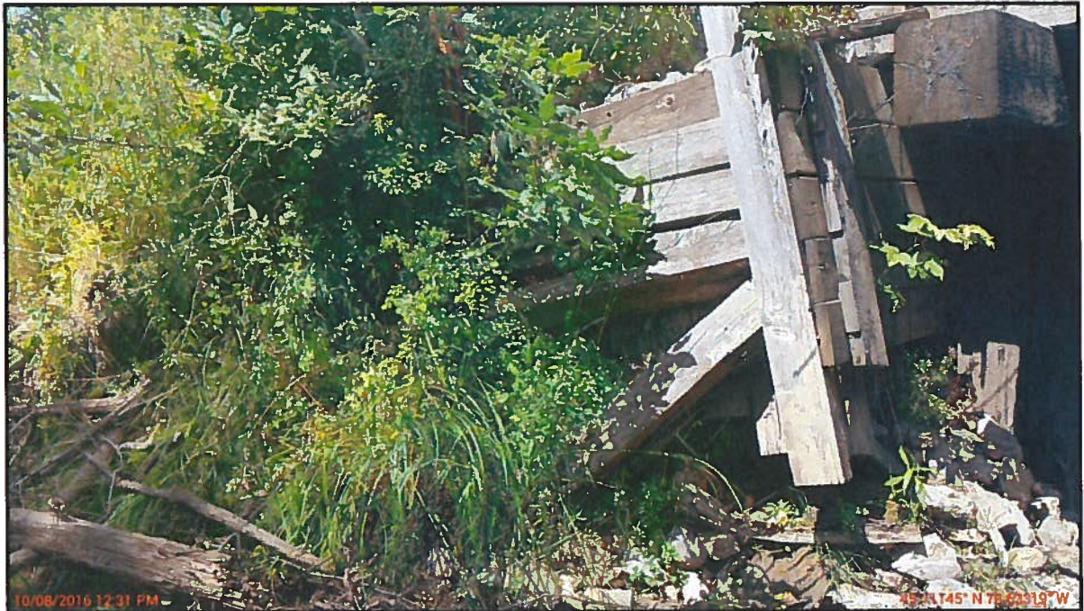
Photo 6: Undermined Ballast Wing Wall – Southwest Quadrant
