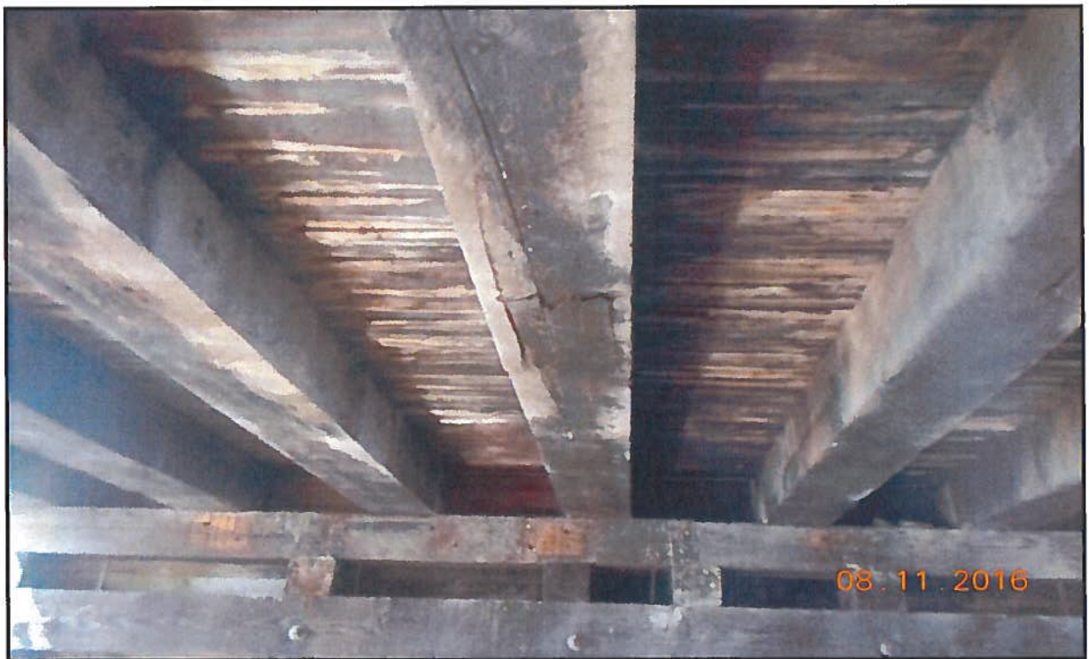
Photo 6: Splintering of Wood Beam (4 th from North face) – Looking West
