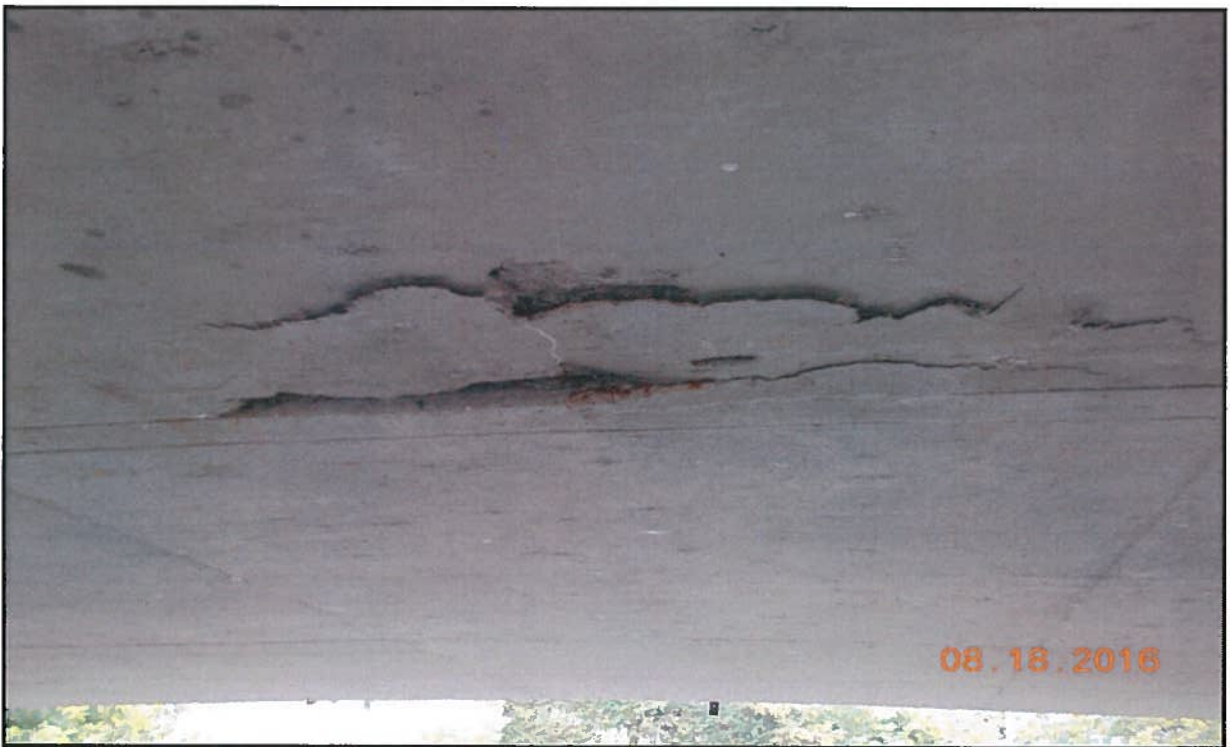
Photo 8 : Spalling Concrete – Mid Span of Soffit Looking East
