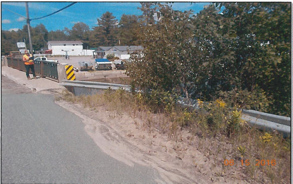
Photo 4 : Deformed Guiderail System Missing Supports - Southeast Quadrant
