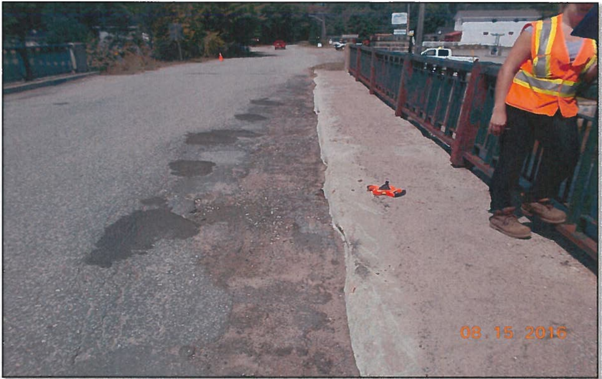
Photo 3 : Asphalt Wearing Surface and Curb Deterioration - East Lane Looking North
