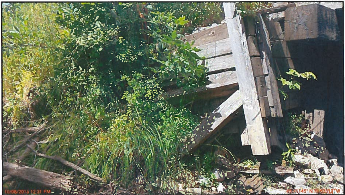
Photo 6: Undermined Ballast Wing Wall – Southwest Quadrant
