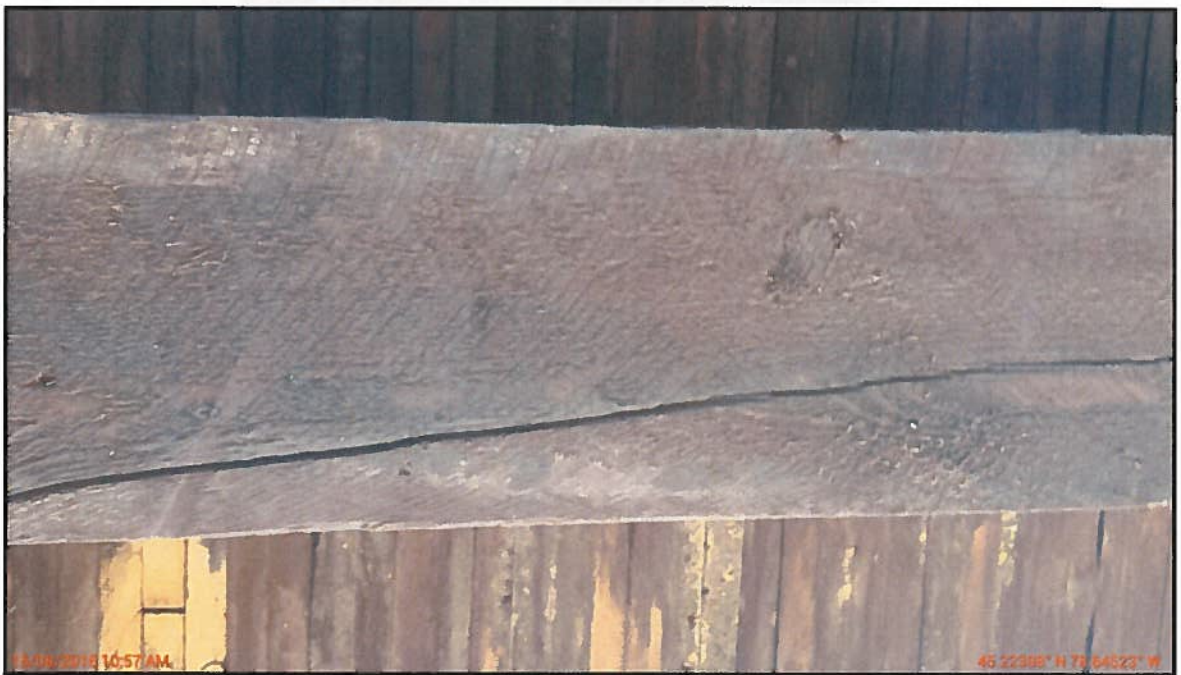
Photo 8: Longitudinal Cracking of Wood Beam (4 th from North face) – Close Up View
