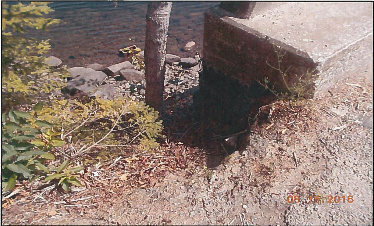
Photo 7 : Erosion of Embankment - Northwest Quadrant
