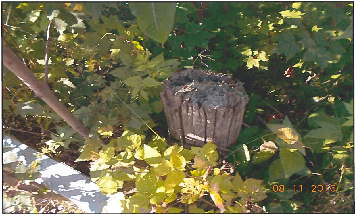
Photo 6 : Typ. Approach Barrier Post with Severe Splits – Southeast Quadrant
