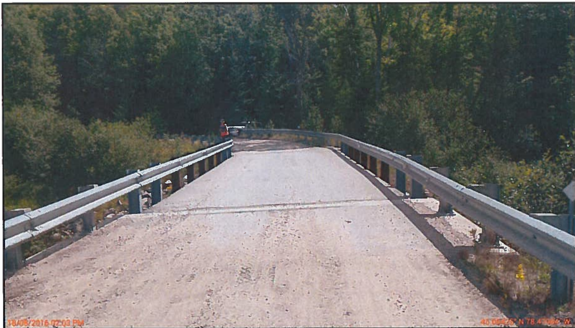
Photo 2 : General Arrangement – Looking South
