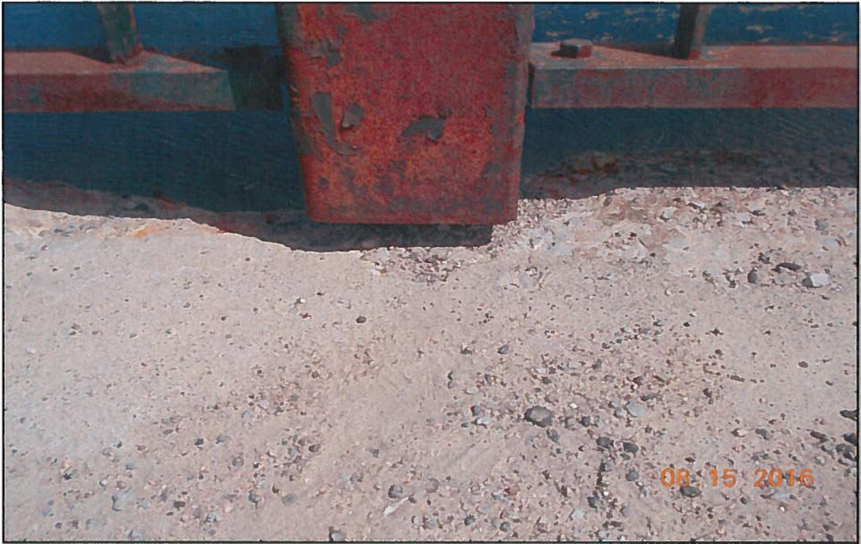
Photo 7 : Inadequate Load Carrying Capacity at Handrail Posts - Typical View
