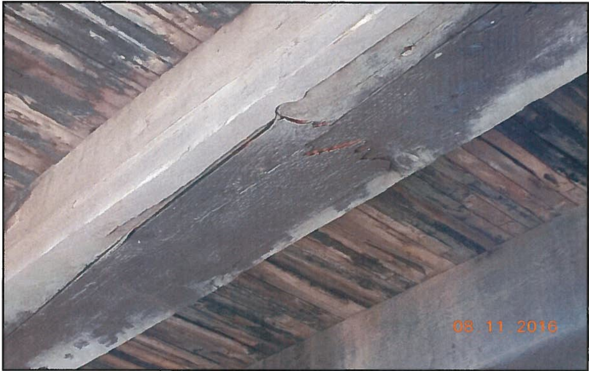
Photo 7: Splintering of Wood Beam (4 th from North face) – Close Up View
