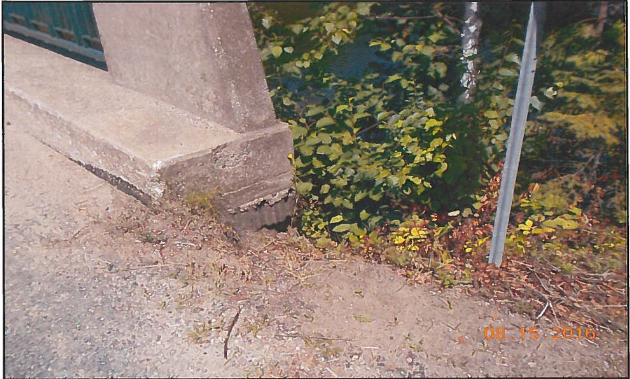
Photo 9 : Erosion of Embankment - Northeast Quadrant
