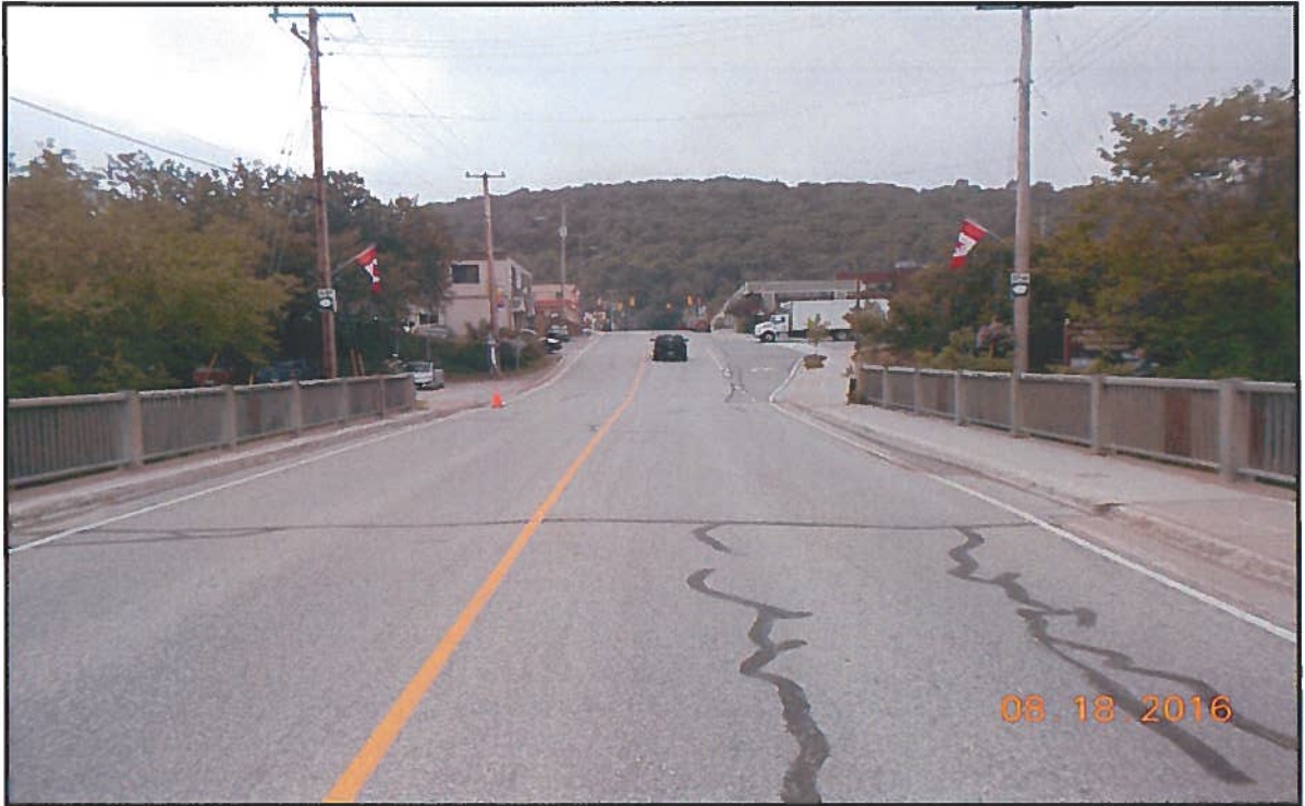
Photo 1 : General Arrangement - Looking South
