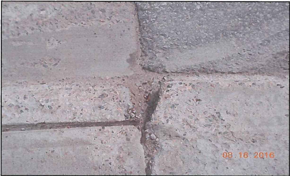
Photo 7 : Curb Deterioration – Southwest Quadrant
