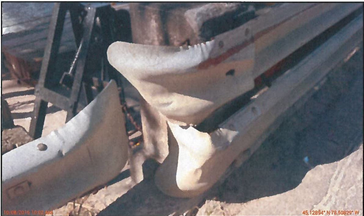
Photo 16 : Damaged Guiderail System – Southwest Quadrant
