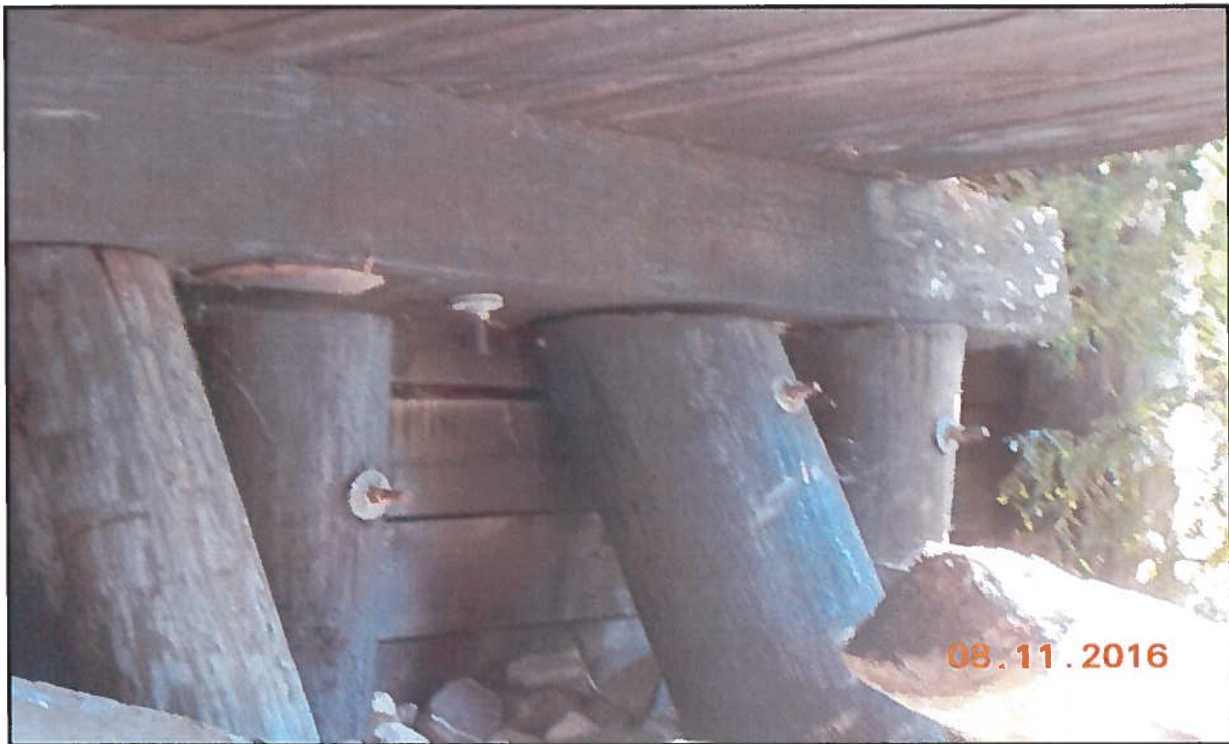
Photo 5 : Gaps Between Piles and Capping Beam – Northeast Quadrant
