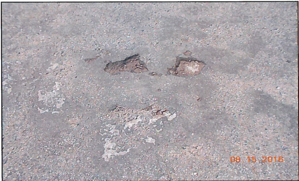
Photo 6 : Deck Wearing Surface - Localized Potholes
