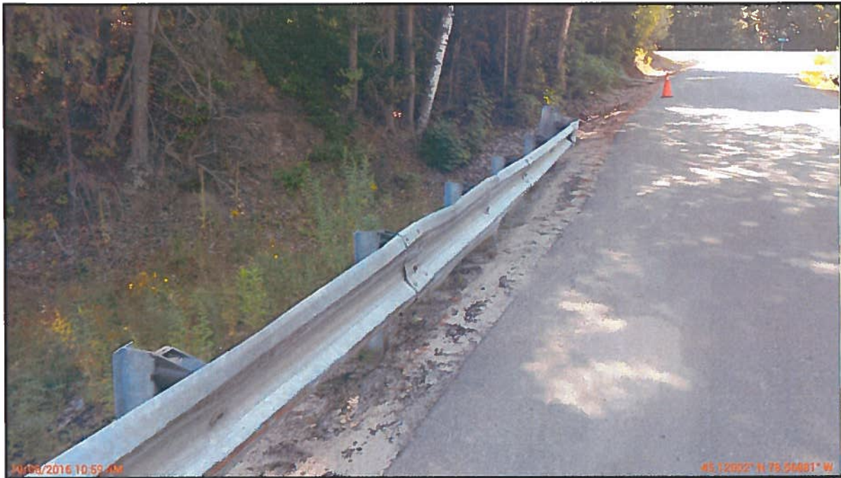
Photo 5 : Guiderrail Impact Damage - Southeast Quadrant
