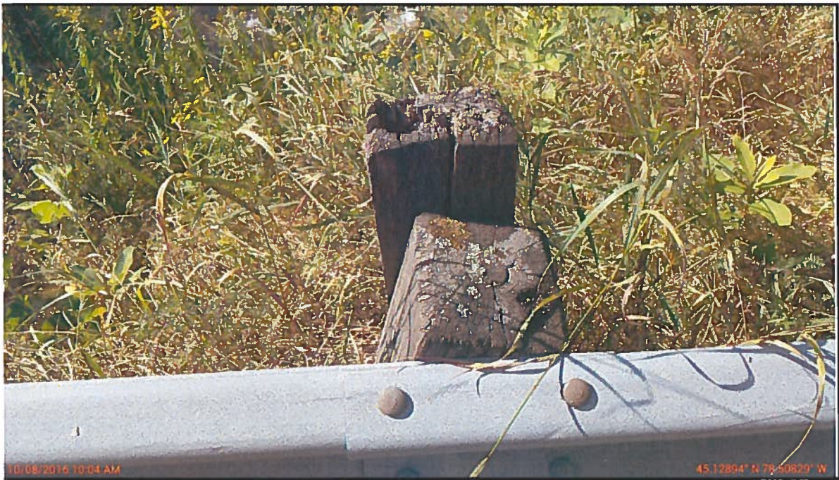
Photo 17 : Typ. Rotted Post – Southwest Quadrant
