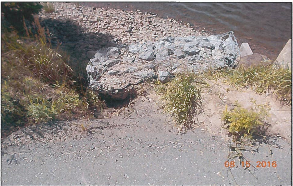
Photo 8 : Erosion at Gabion Basket Retaining Wall - Southwest Quadrant
