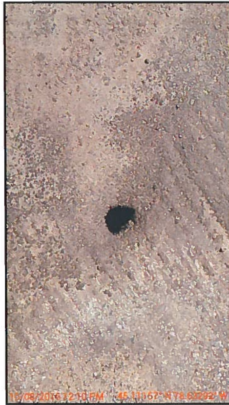
Photo 5: East Approach Wearing Surface – Undermined Asphalt Zone (Sinkhole)
