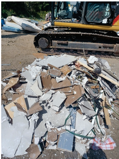
Figure 3.3 Drywall from the August 12th CND Pile
