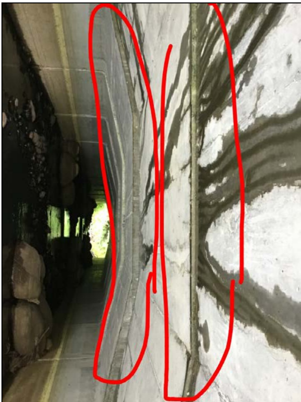
Description: Seepage, through furthest 2 section joints to the north Culverts / Barrels
