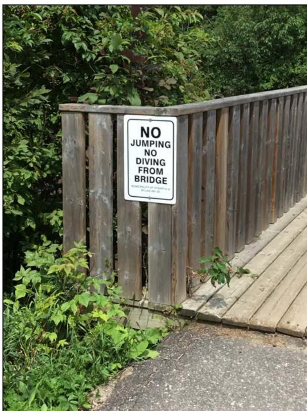
Description: Warning sign, south side. Accessories / Signs (N/S)
