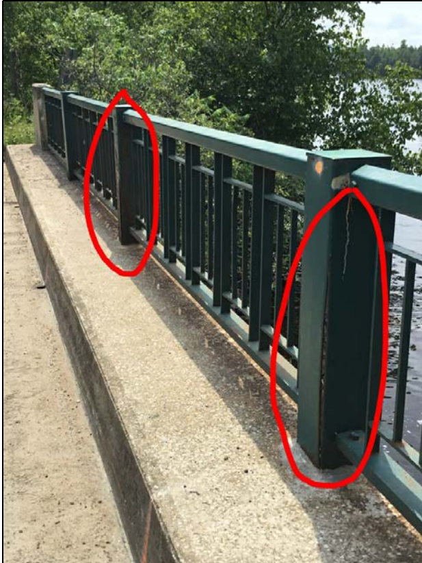
Description: Cracking of both centre posts on south side Barriers / Hand Railings (North and South)
