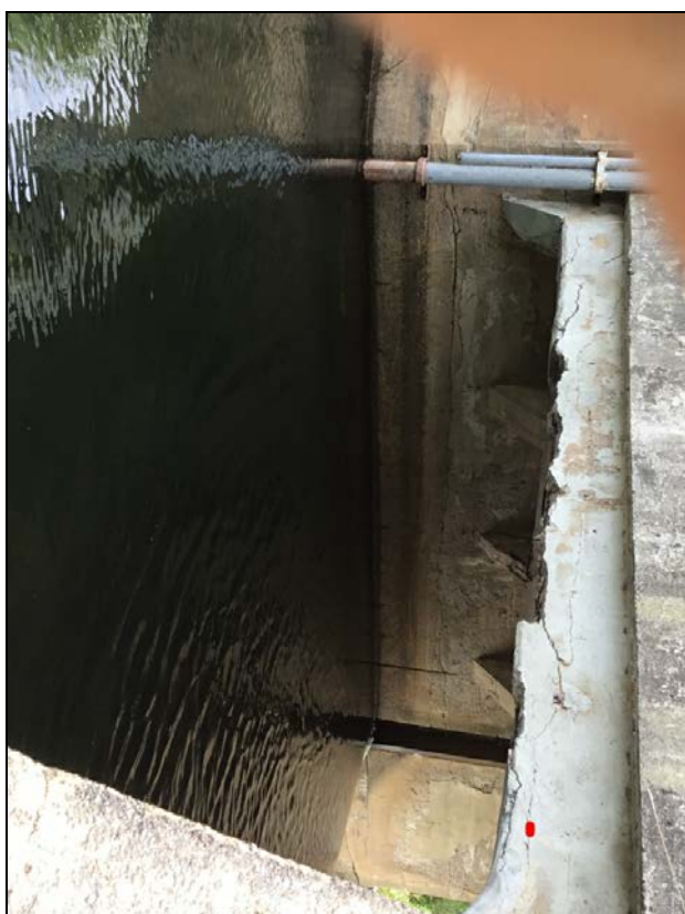
Description: East abutment, medium transverse crack at high waterline midway up abutment wall.
