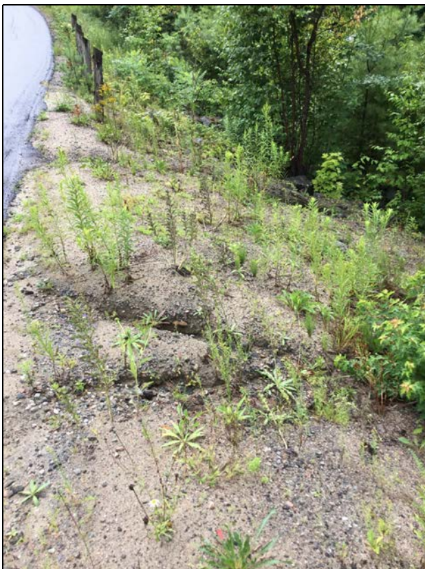
Description: Northwest erosion \ washout detail.
