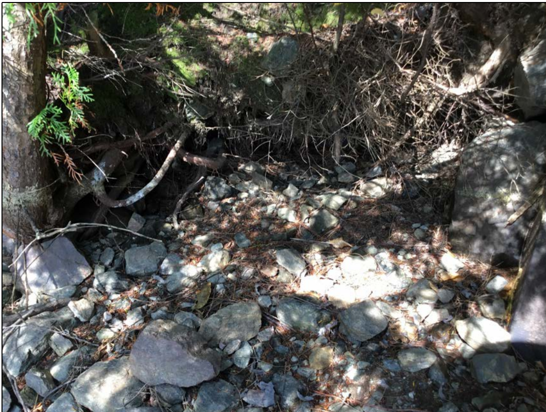
Description: Undermining at high water mark with overlaying root mat at northwest quadrant.
