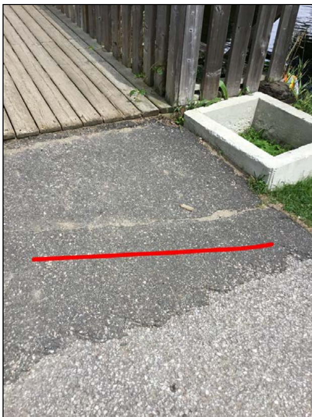
Description: Crack in asphalt access ramp. Approaches / Sidewalk/Curbs (South only.)
