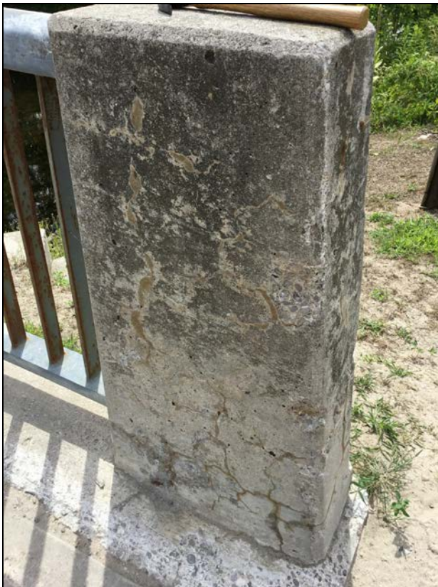
Description: Light map cracking at northwest parapet.
