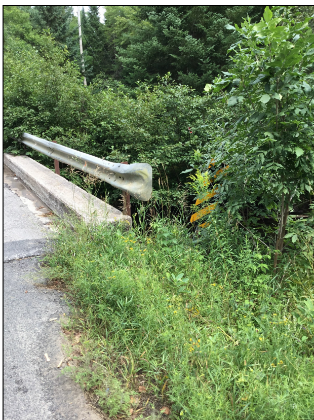
Description: SW hazard is bent obstructed by vegetation.
