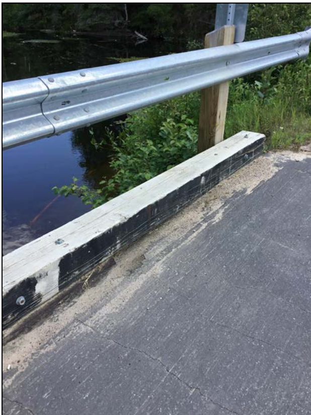
Description: New curb at northeast corner. Bolts are not countersunk. Sidewalks/Curb / Curb (N /S)
