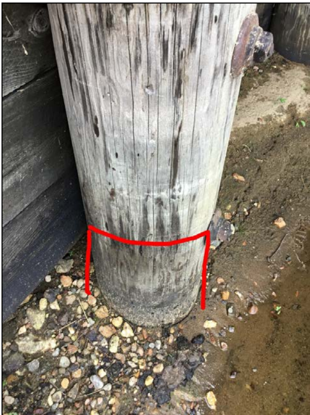
Description: Typical area of minor rot, south side.
