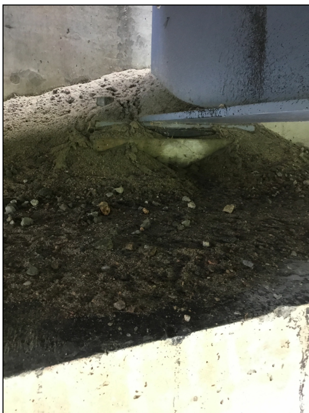
Description: South wall, sediment is washing down from above and accumulating around the bearing on the bearing seat from a defective joint fill above.
