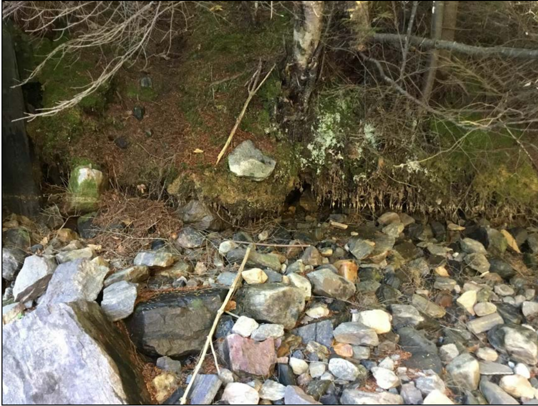
Description: Undermining at northeast Embankments & Streams / Embankments
