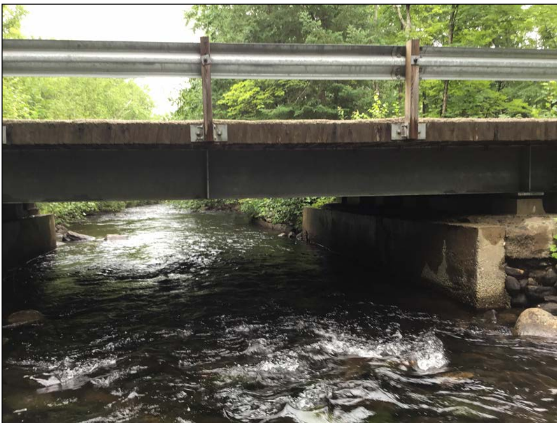
Description: West exterior soffit, slight deflection and movement of deck boards visible.
