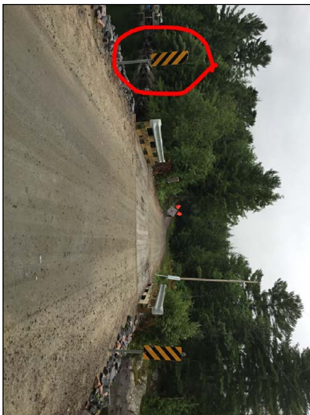
Description: SE hazard damaged, Accessories / Signs
