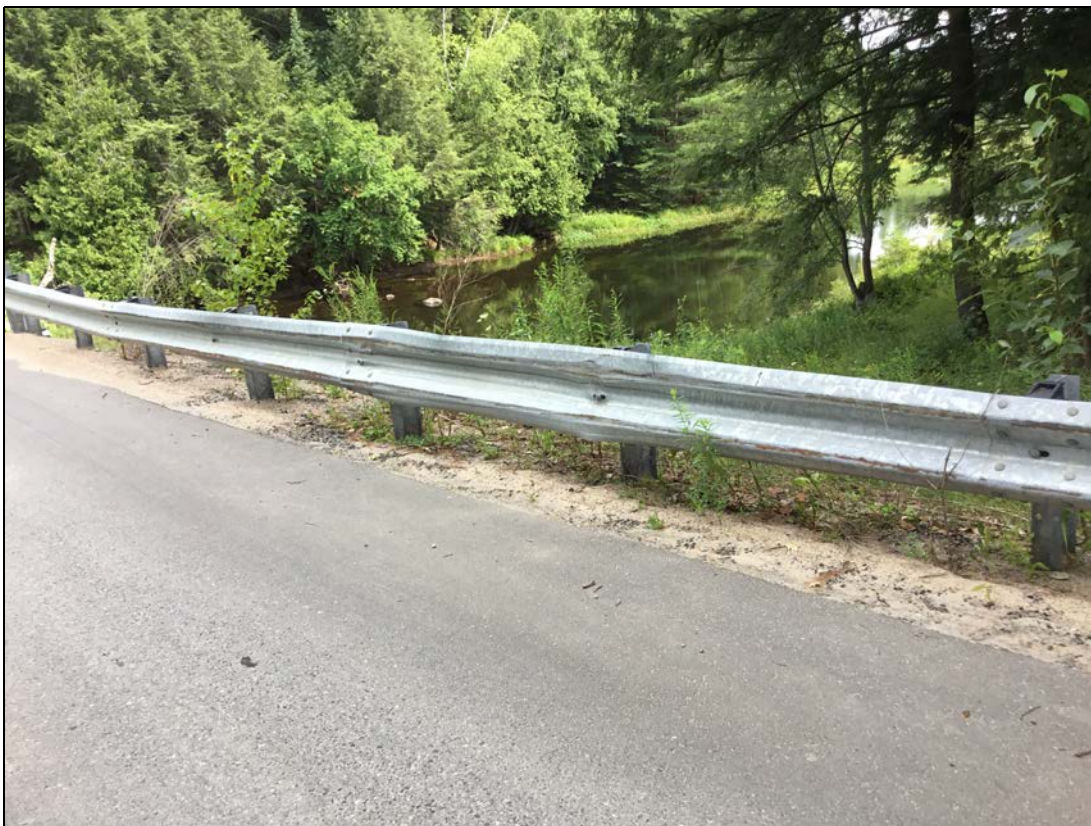
Description: SW rails have impact damage Barriers / Railing Systems (E/W)
