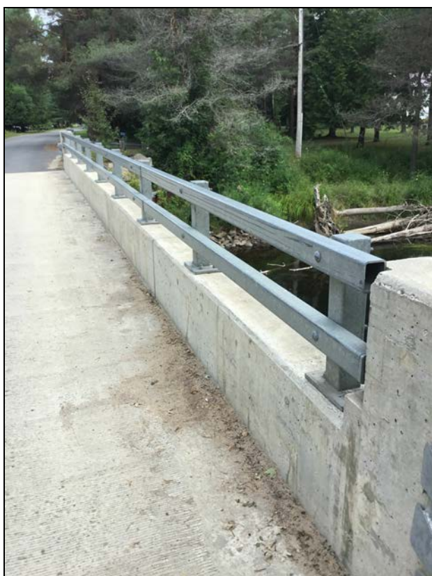
Description: East handrail, Impact scraps of handrails causing light corrosion Barriers / Hand Railings (E/W)
