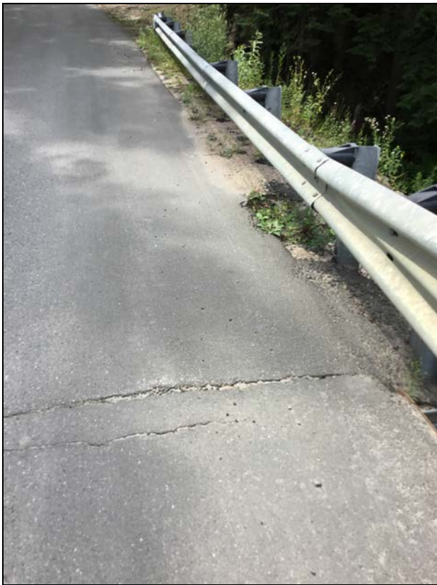
Description: SW erosion / cracking Approaches / Wearing surface (N/S)
