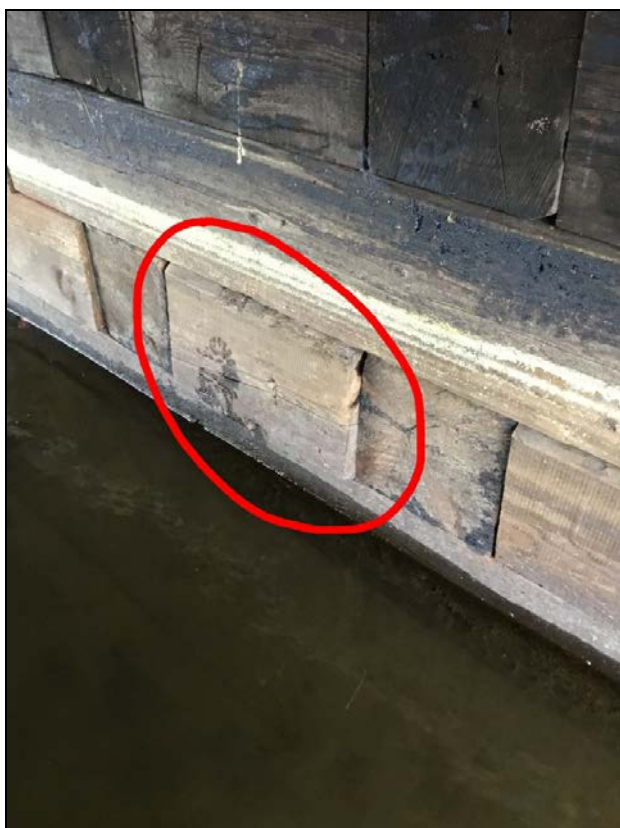
Description: West abutment midspan, shaken, split and loose Abutments / Abutment Walls
