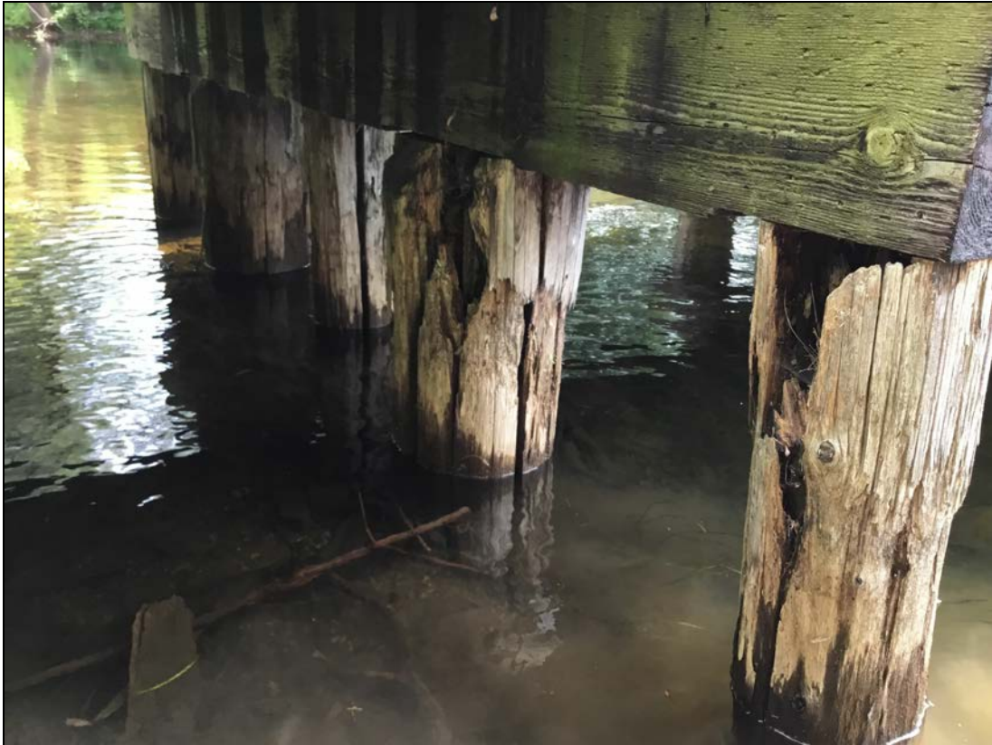
Description: Second to north piers looking, looking southeast. Severe disintegration. Piers / Shafts/columns/Pile Bents
